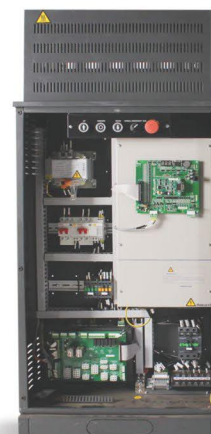
Integrated Control Panel
