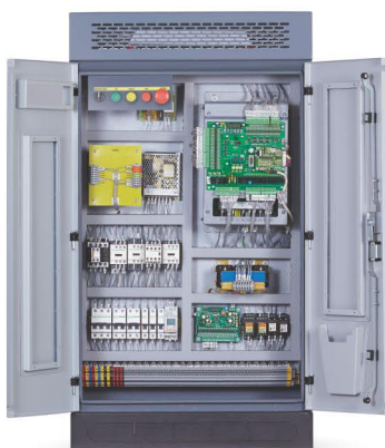
Integrated Lift Controller AS 360 Parallel Type
